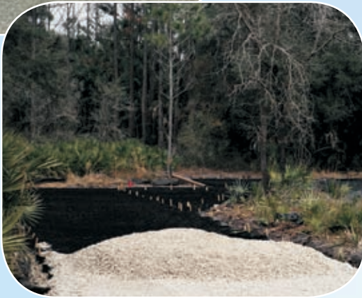
Preparing the base by placing a geotextile fabric over the muck soil. Next, Geoweb sections were placed over the geotextile fabric, staked and infilled with #57 stone.
